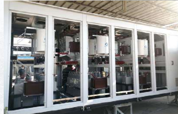
66/11kV GIS 9 MvAR Capacitor Bank Egyptian Electricity Transmission Co.
